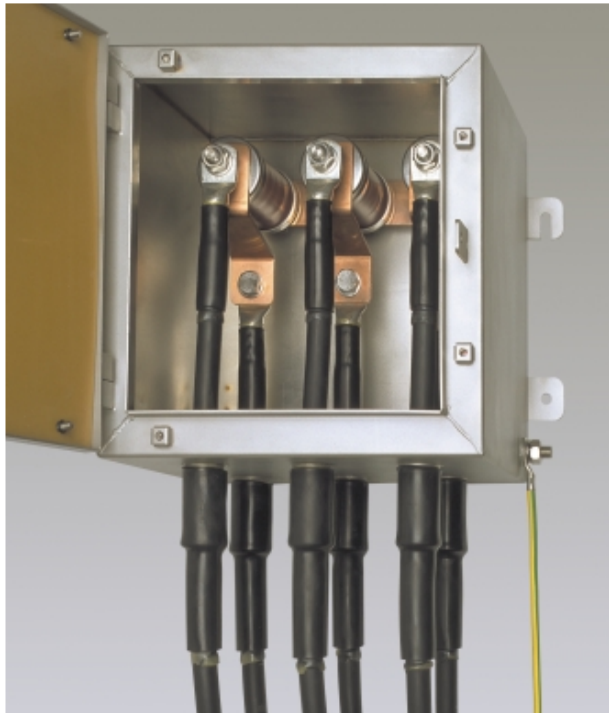
Link box installed with cross bonding cables
